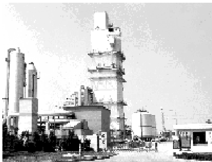
4200 tpd oxygen plant No. 6 at Baoshan Iron & Steel (Group) Corp. of Shanghai was built with mostly Chinese manufactured parts and equipment.
